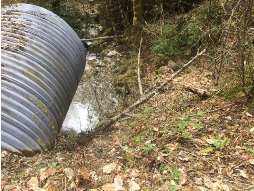
Right bank outlet erosion
