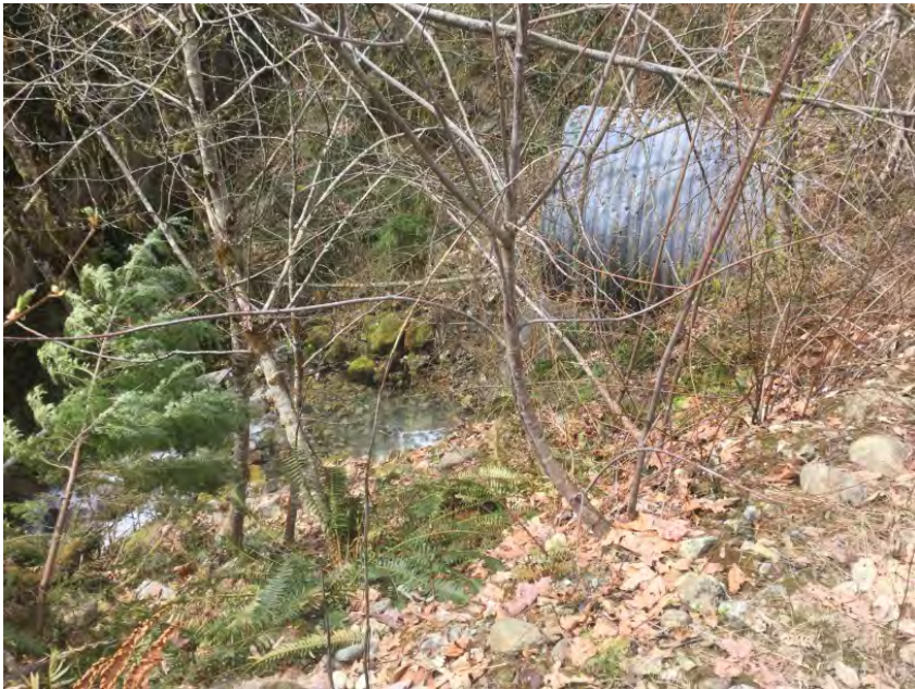
Left bank outlet erosion
